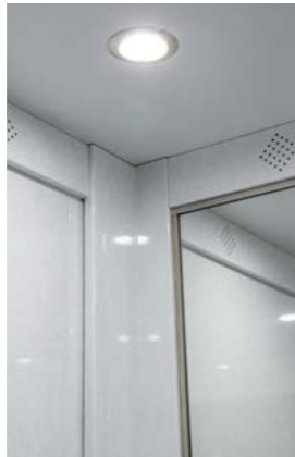
LIGHTING: HIGH EFFICIENCY LED SPOTS
